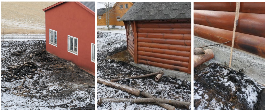
Figure A21. Photos of building 6d (left), garden grill cottage 6c (middle and right). Photos: RISE Fire Research.
