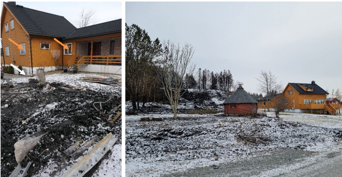
Figure A18. Photo taken standing at garage 6a towards house 6b (left). Two cracked windows are marked by orange arrows, and charring on the ground by a white arrow. Photo taken standing on the road towards garden grill cottage 6c and house 6b (right). Photos by RISE Fire Research.
