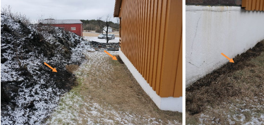
Figure A19. Photo behind house 6b looking towards garage 6a (left). Arrow marks surface charring. Close-up photo of the charring of the narrow strip of grass litter against the foundation (right). Photos by RISE Fire Research.
